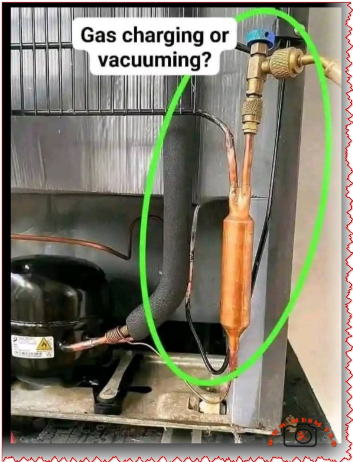
Gas Charging or Vacuuming? Understanding the Service Valve on Small Refrigeration Units
