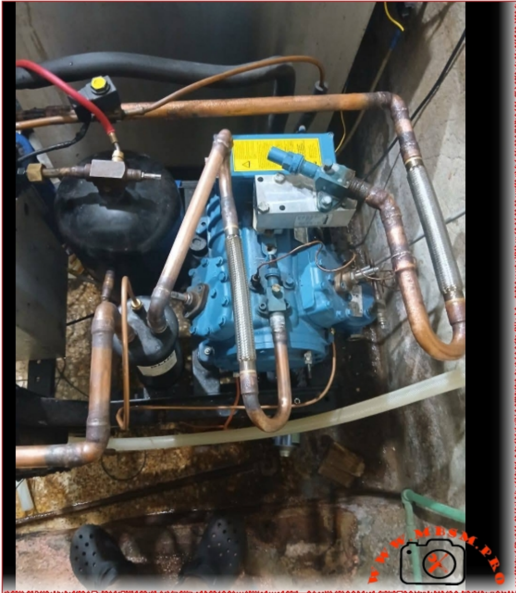
Best piping practices for semi-hermetic systems mbsmpro
